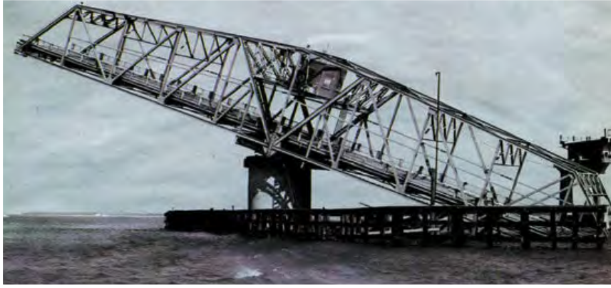
Sgt. Price was “in a state of shock” when he saw the Ben Sawyer Bridge, which connects Sullivan’s Island to Mount Pleasant, dangling in the Intracoastal Waterway.
