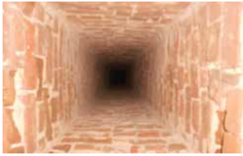
The kiln at Brickyard plantation, looking up from the inside. Photo by Hope Rechea.
