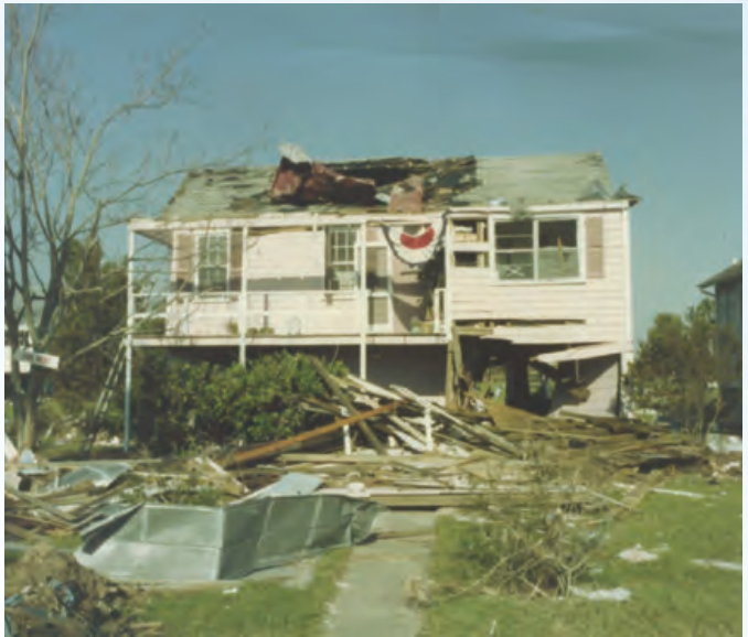
Many homes in the Lowcountry suffered severe roof damage during Hugo's trip through the area.
